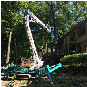
Expensive and complex equipment is often needed around homes.
